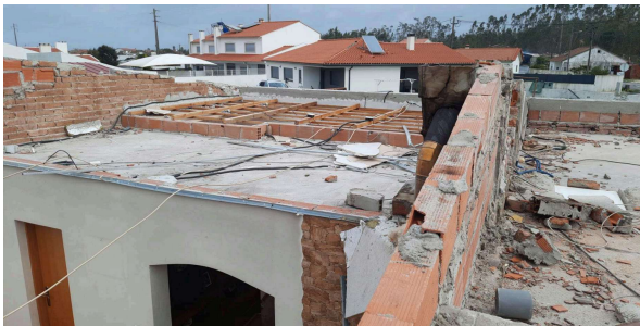
Home damaged by Storm Kristin
